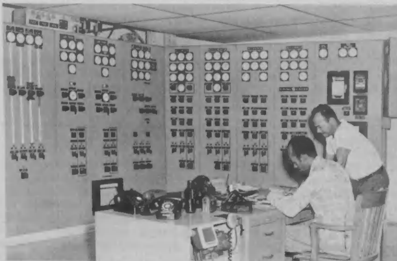
INTERIOR VIEW of Powerhouse No. 1 panel enclosure, with operator's desk and part of panel. VISTA INTERIOR di cuarto rond di panel den Powerhouse No. 1, cu lessenaar di operador y parti di panel di control.
